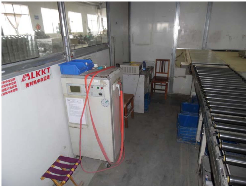
Fan coil run test room to check fan speed ,noise, electric insulation ,electrical leakage etc
